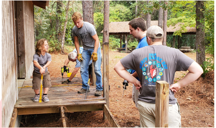
L to R: Ian Bankester, Connor Simms, Austin Kelsey, and Addison Broom working on the ramps at Camp Hobbs
